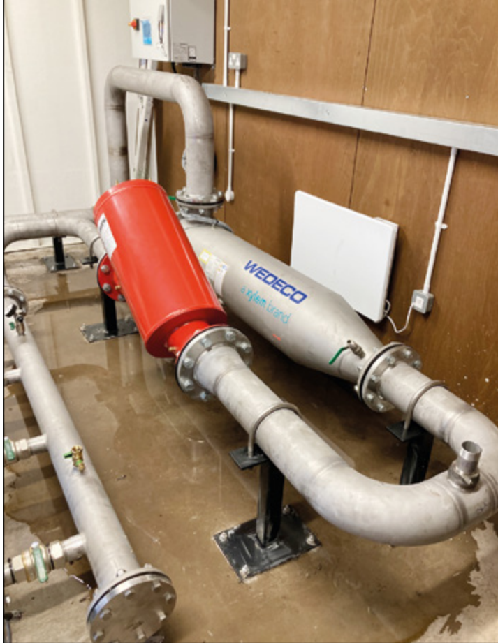
Ultra Violet Water Treatment
