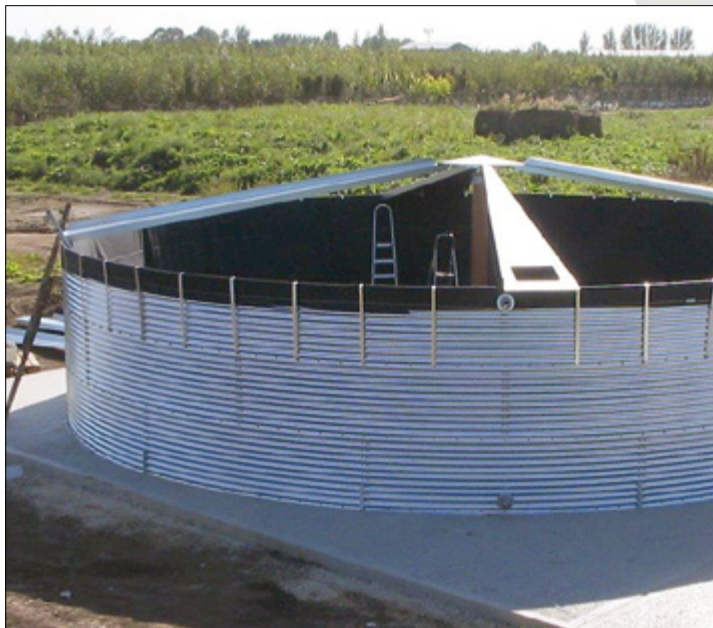
Water storage tank installations
